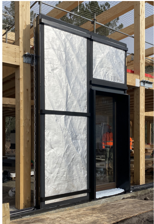
FIG. 3 Basajaun's curtain wall modules' inner part installed on construction site. (credit: Basajaun H2020, picture by Vandi, L.)
